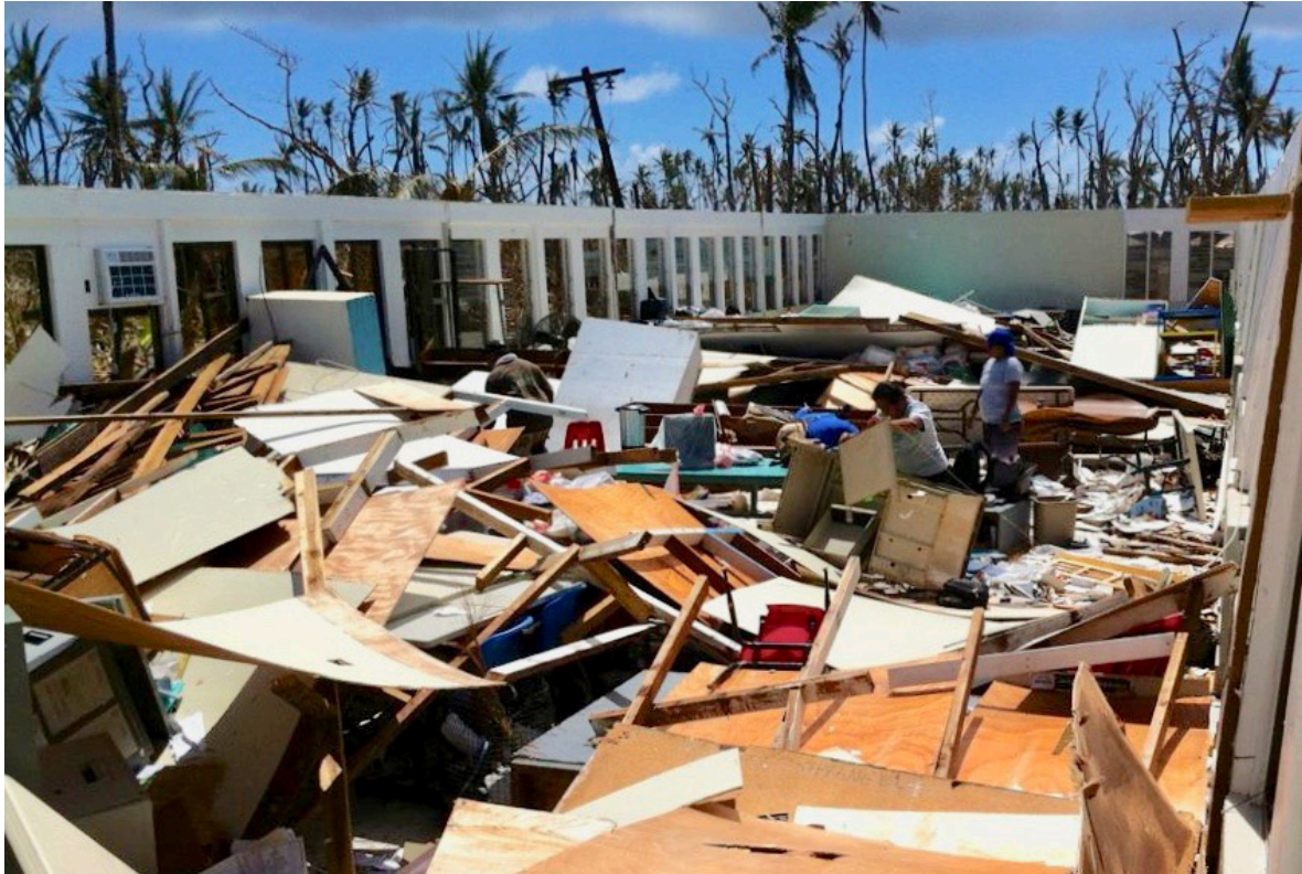
During Typhoon Haiyan in 2013, high winds heavily damaged public schools in Kayangel, as shown here. The year before, educational facilities on the east side of Babeldaob were flooded during a storm surge caused by Typhoon Bopha. Photo: Palau Ministry of Education.
